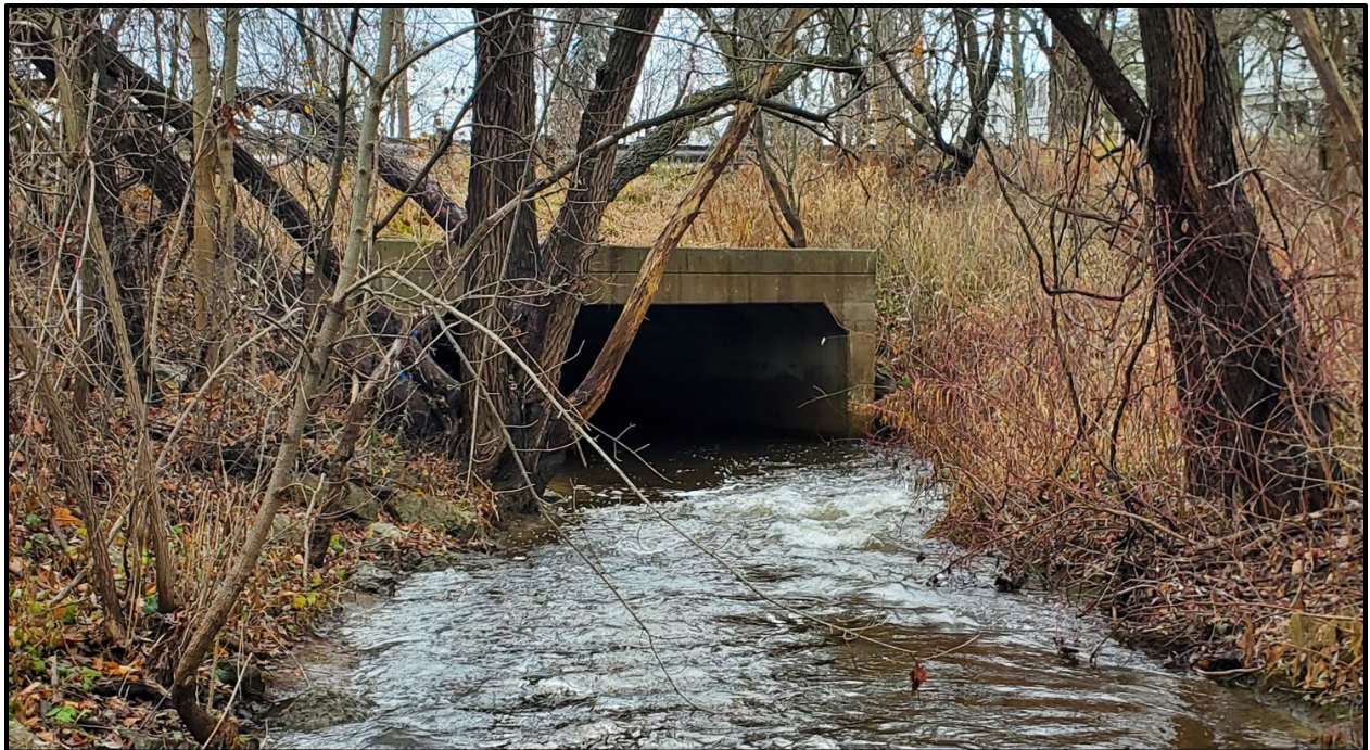
Figure 5-6: Elevation View on Upstream Side of Main Street Concrete Open Footing Box Culvert
