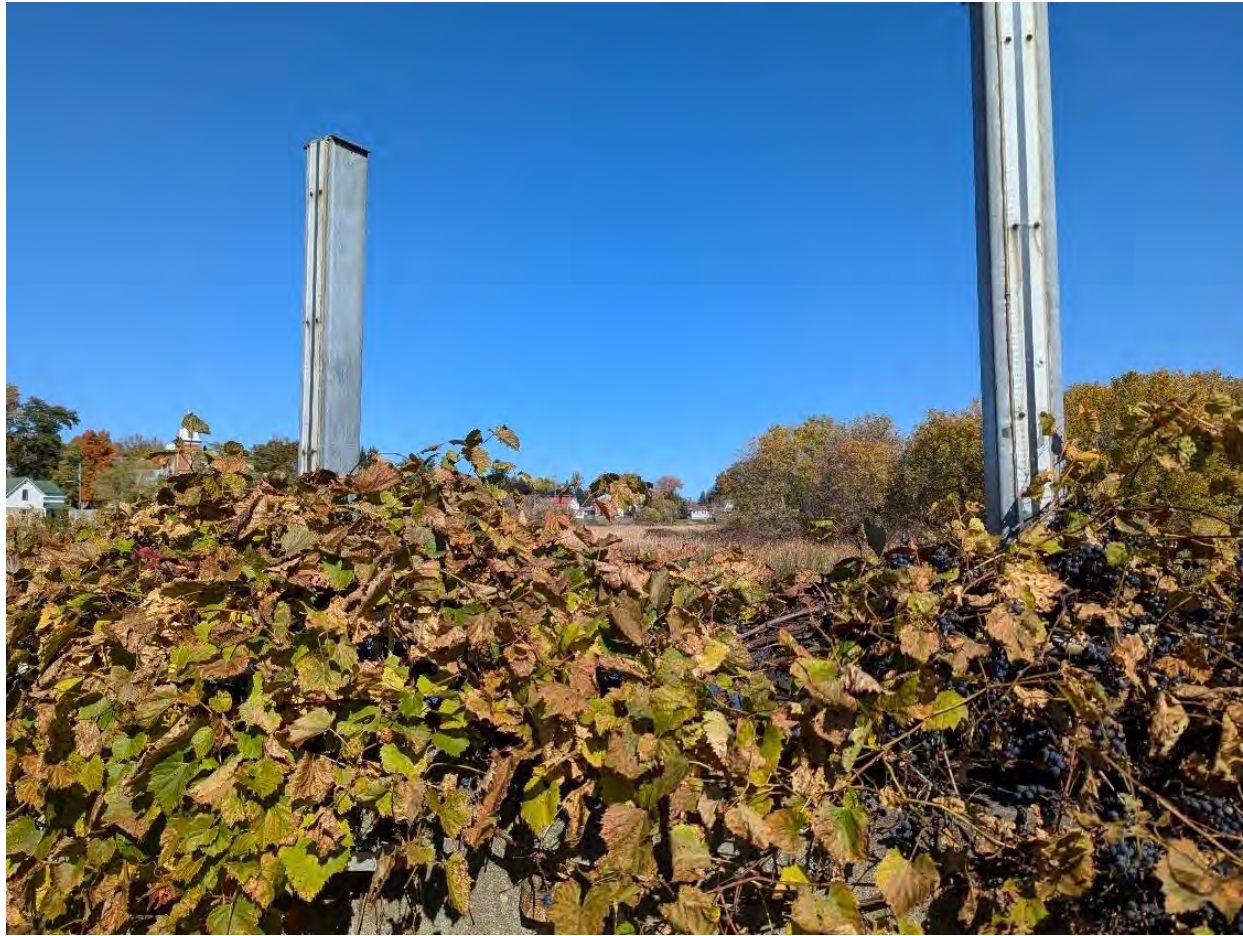
Figure 40: Vegetation impeding the gate opening
