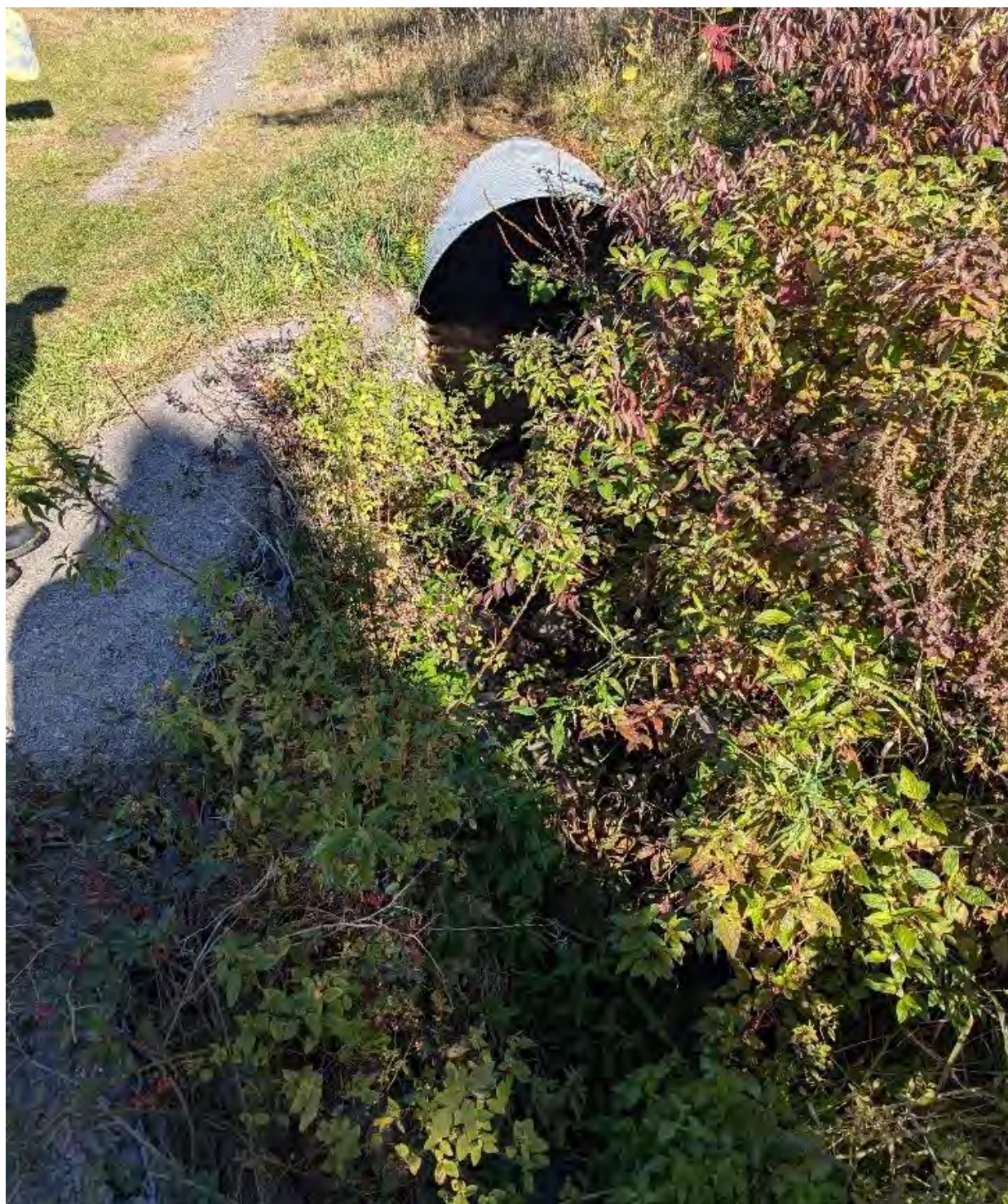
Figure 12: Byron Street – heavy vegetation downstream of culvert
