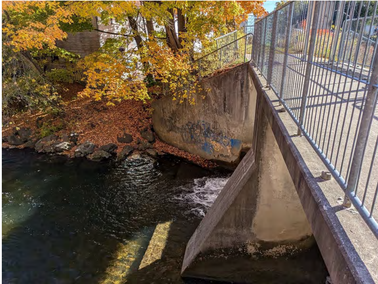
Figure 4: Southern wing wall downstream of dam. Shows location of large tree encroaching towards wing wall
