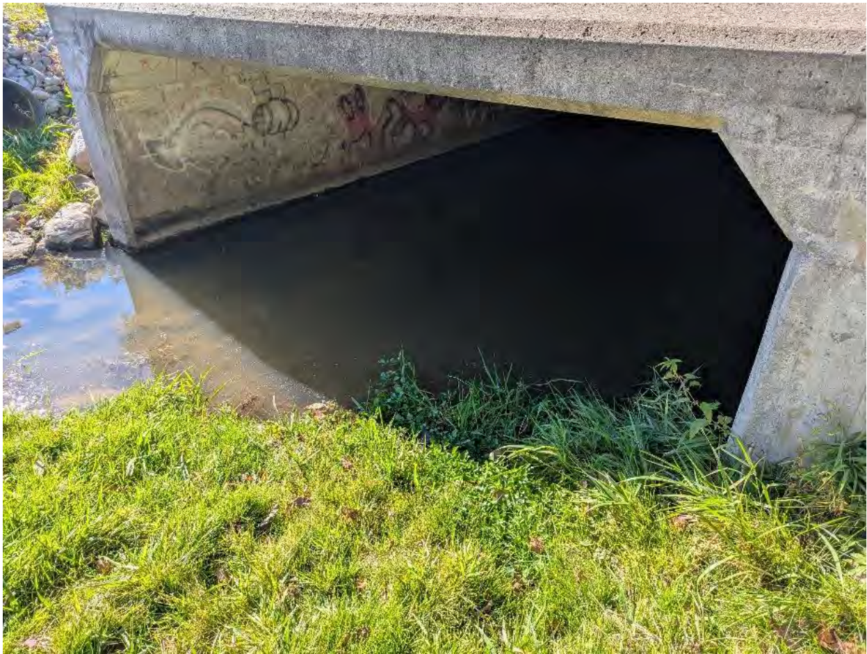
Figure 16: Sediment build-up on the east side of box culvert at Peterson Street
