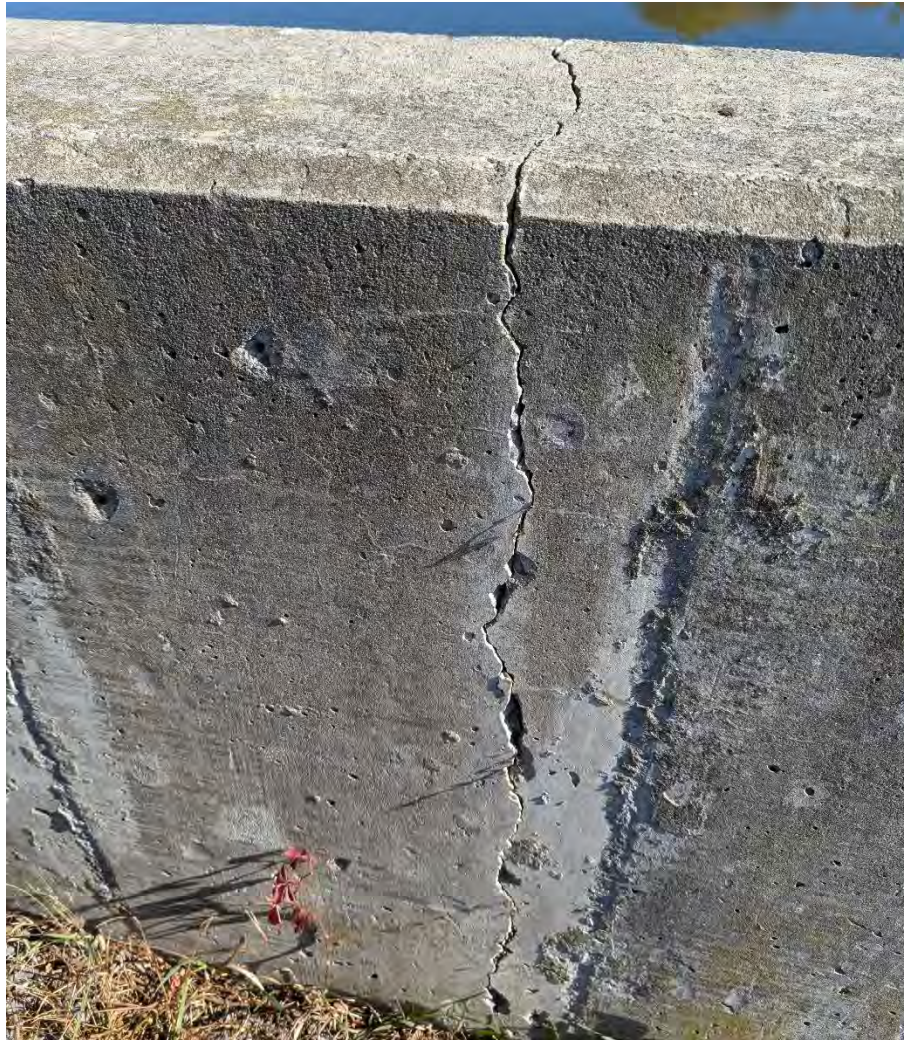
Figure 39: Cracks in concrete flood wall adjacent to Mill Street upstream of weir
