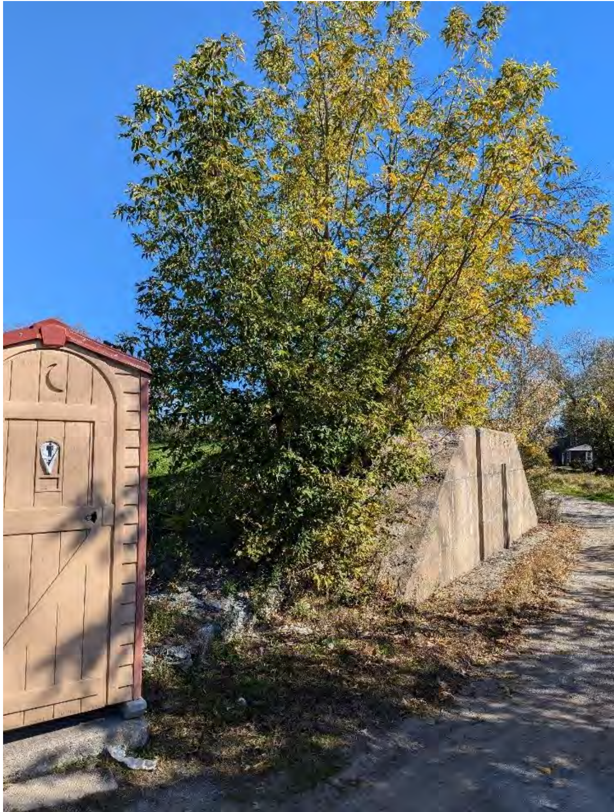
Figure 11: Woody vegetation growth on west side of spillway opening to golf course
