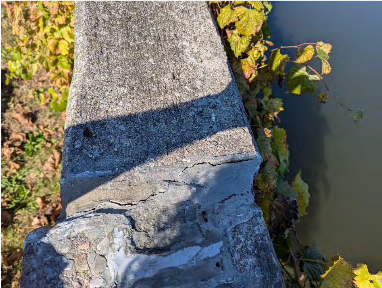
Figure 38: Additional Repaired spalling on wall remaining unchanged since last inspection in 2023
