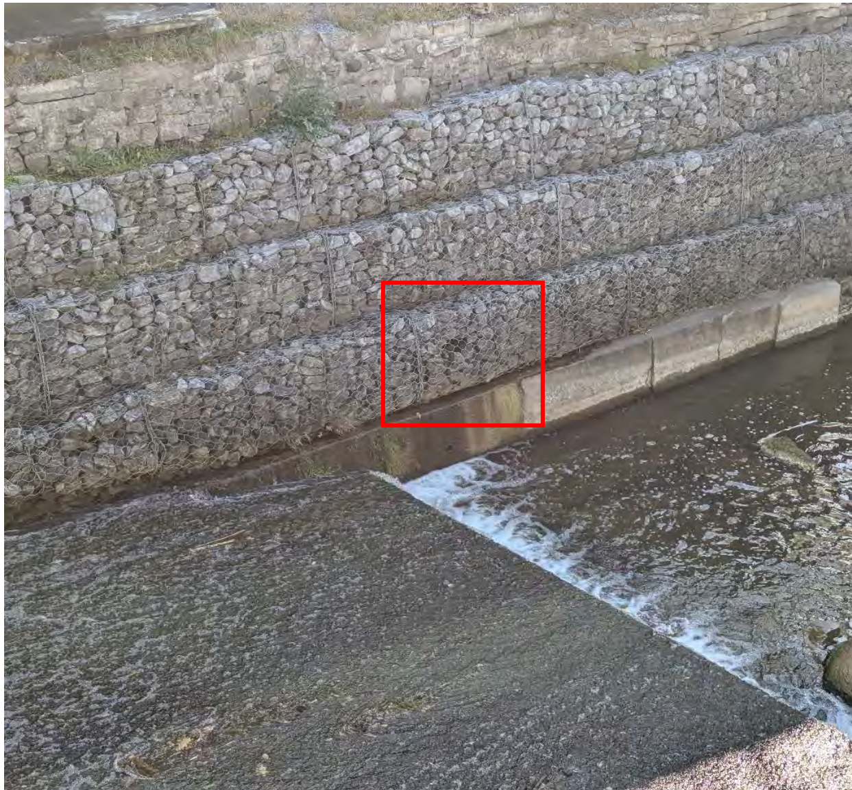
Figure 35: Missing stone from gabion basket on south side of channel near weir dam near 29 James Street
