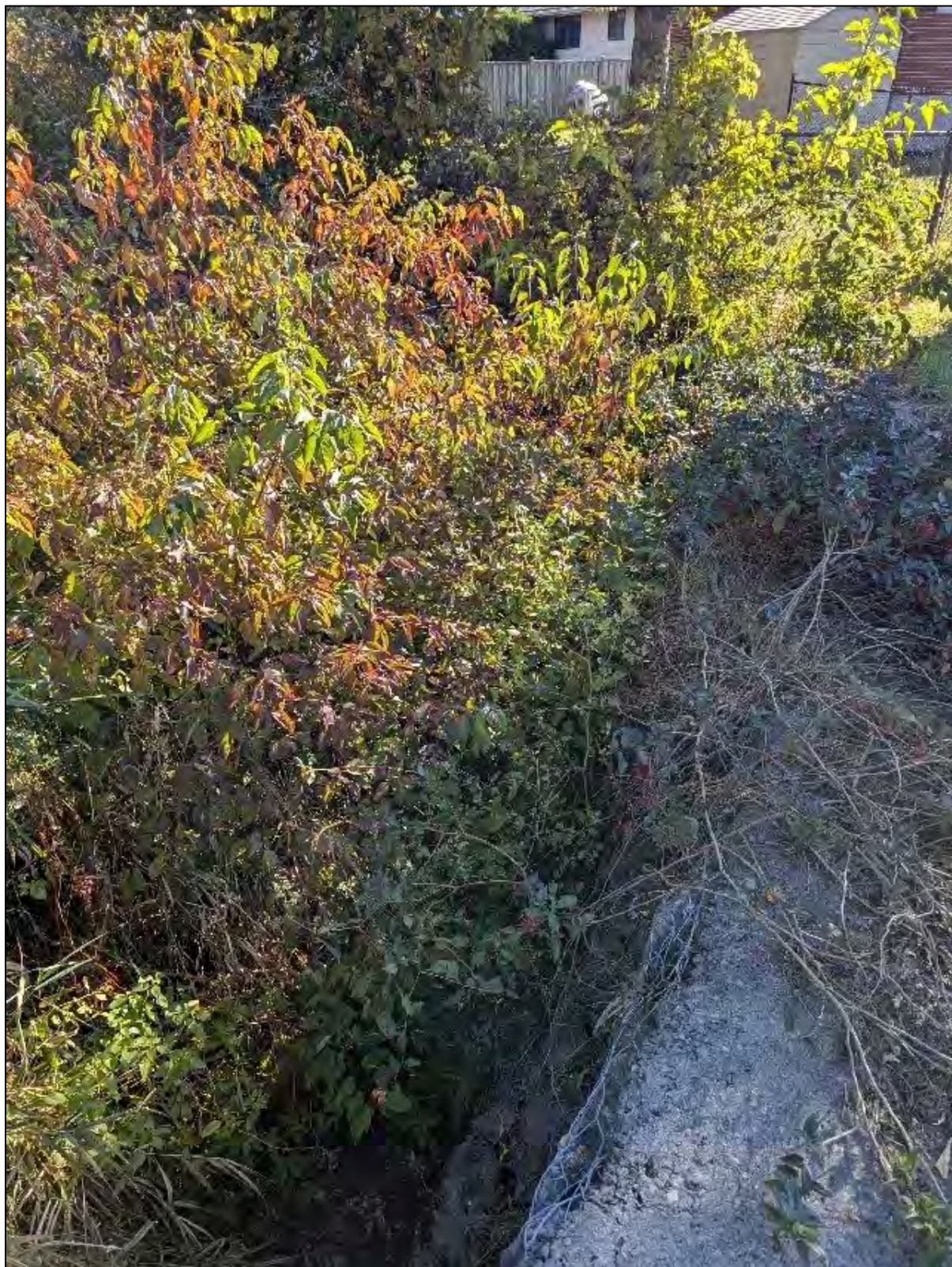
Figure 13: Byron Street – heavy vegetation downstream of culvert
