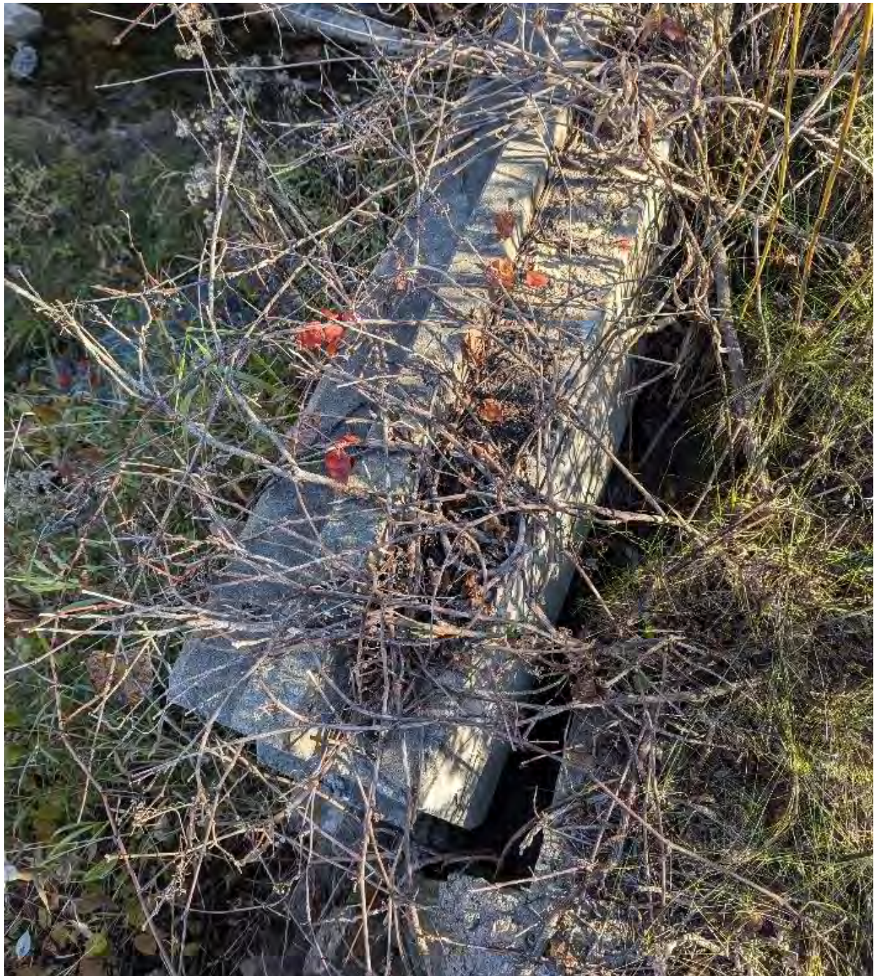
Figure 26: Wing wall on south side of channel on south side of Wooler Road downstream of Double Arch Culvert showing separation
