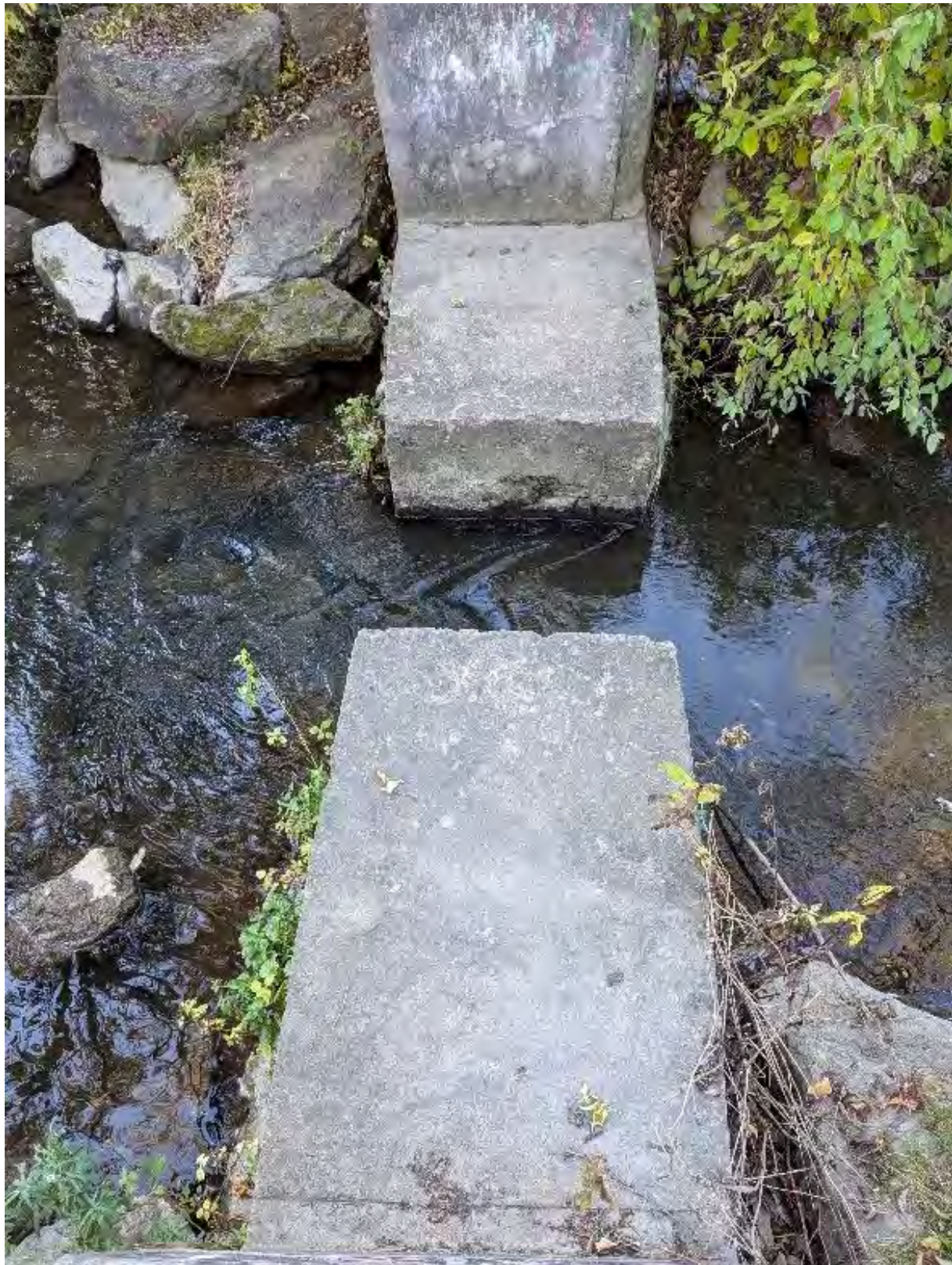
Figure 29:2 stage weir showing some spalling on south side
