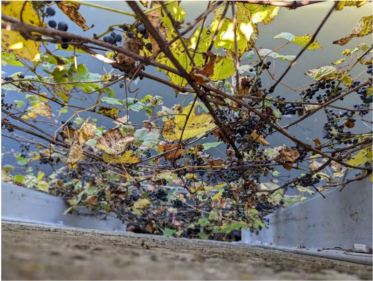
Figure 41: Vegetation impeding the gate operation, top down view
