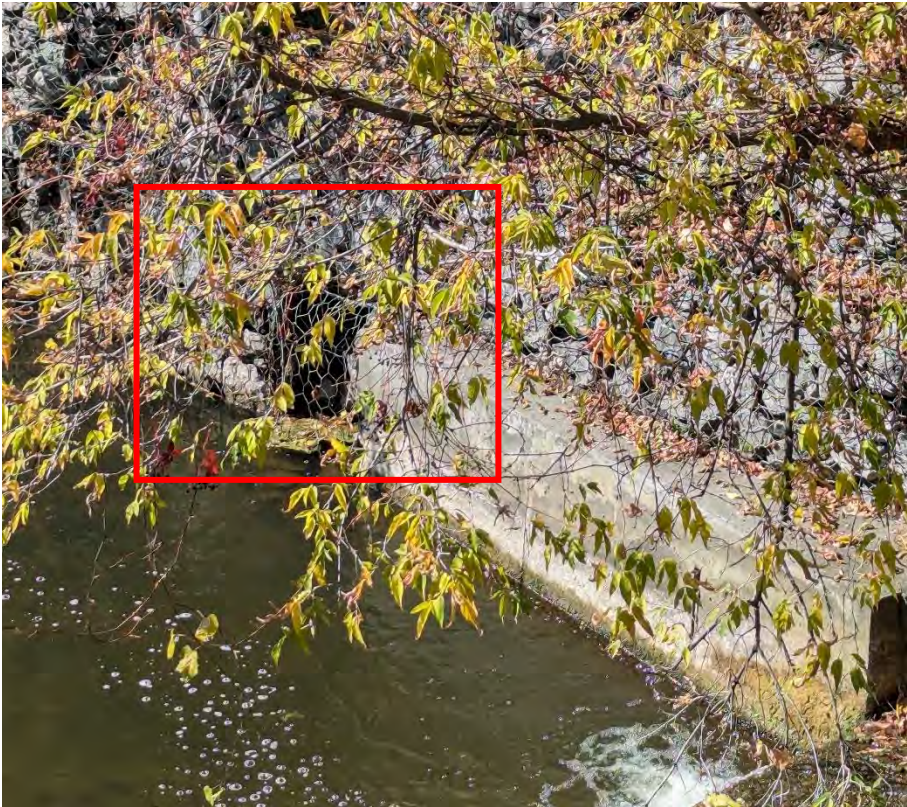
Figure 36: Missing stones from gabion basket on the north side of channel near weir dam near 49 Mill Street
