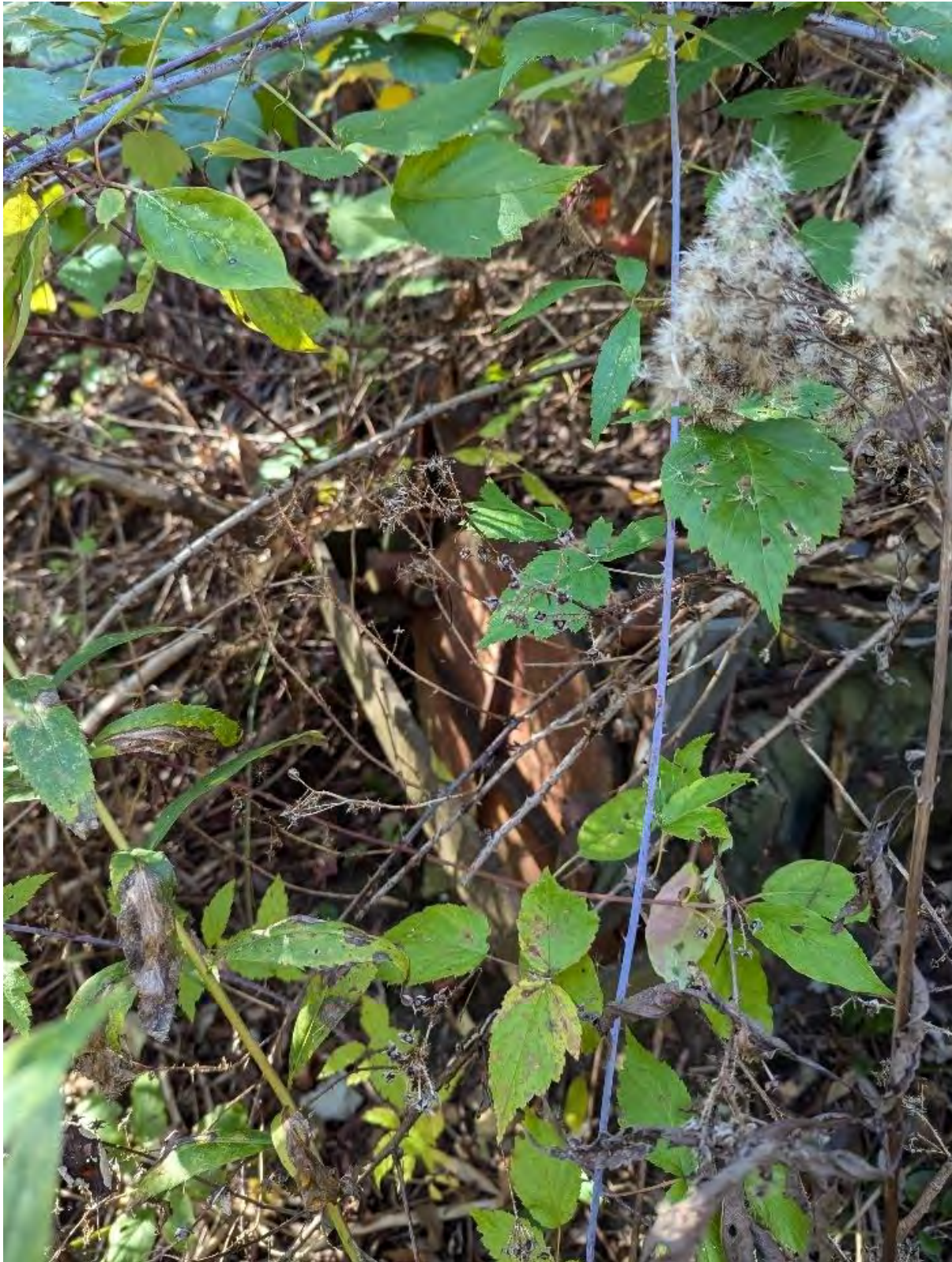
Figure 20: Clear flap gate 2 along Douglas Road berm
