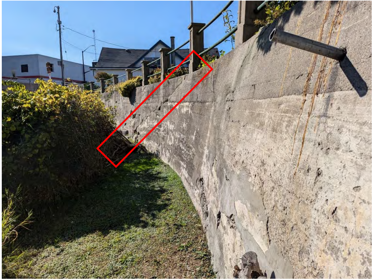
Figure 33: Cracks identified on north side of channel downstream of covered bridge
