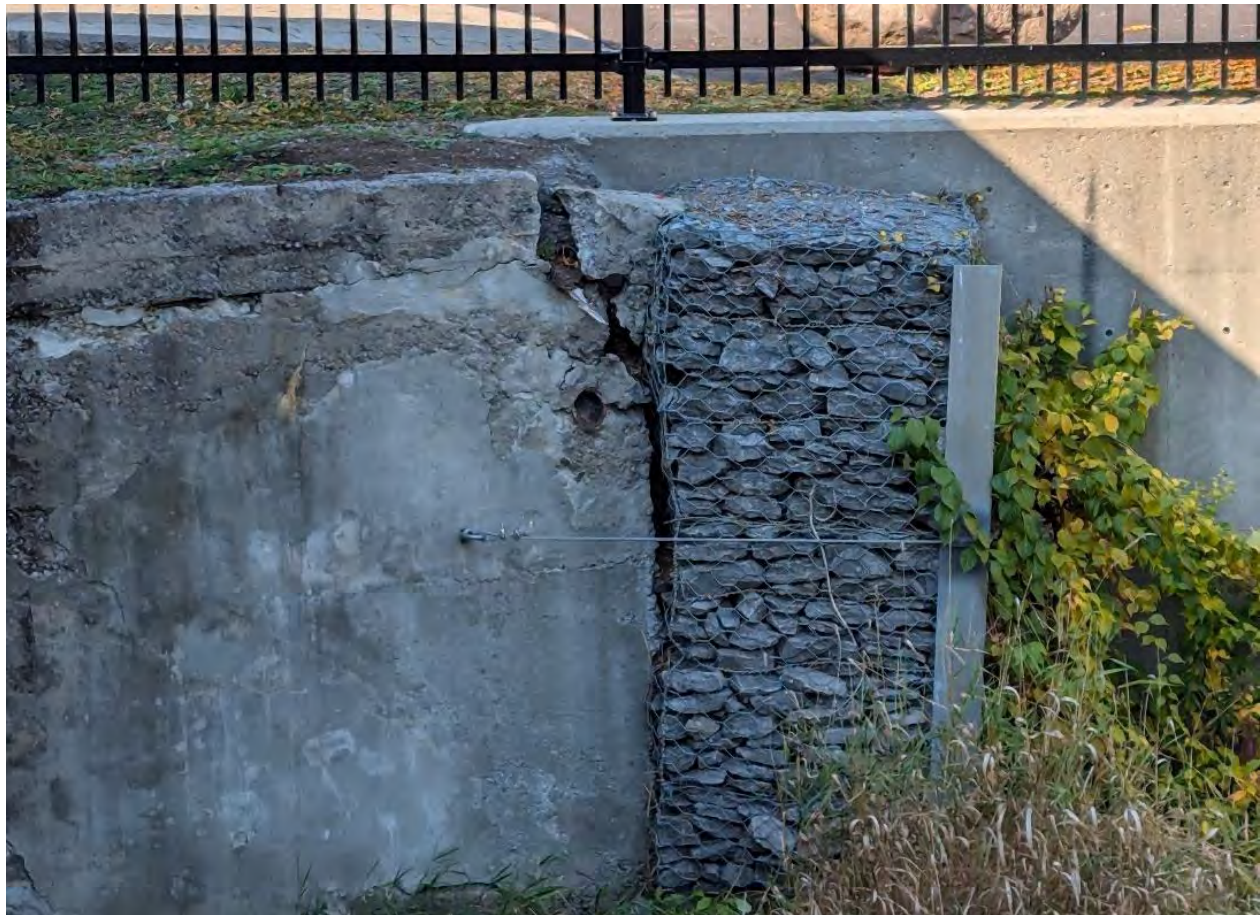
Figure 34: Repair work related to the gabion baskets pulling away from the concrete on the north side of the covered bridge. No change from 2023 inspection
