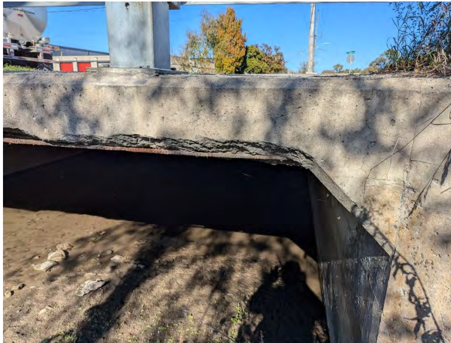
Figure 23/28: Spalling concrete corrosion on Douglas Road culvert
