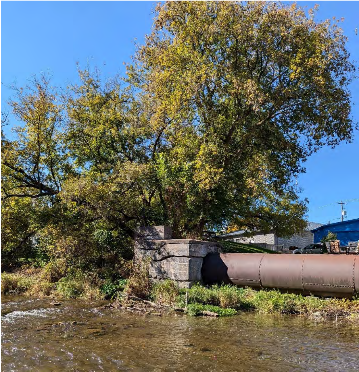
Figure 6: Trees and minor erosion along pipe
