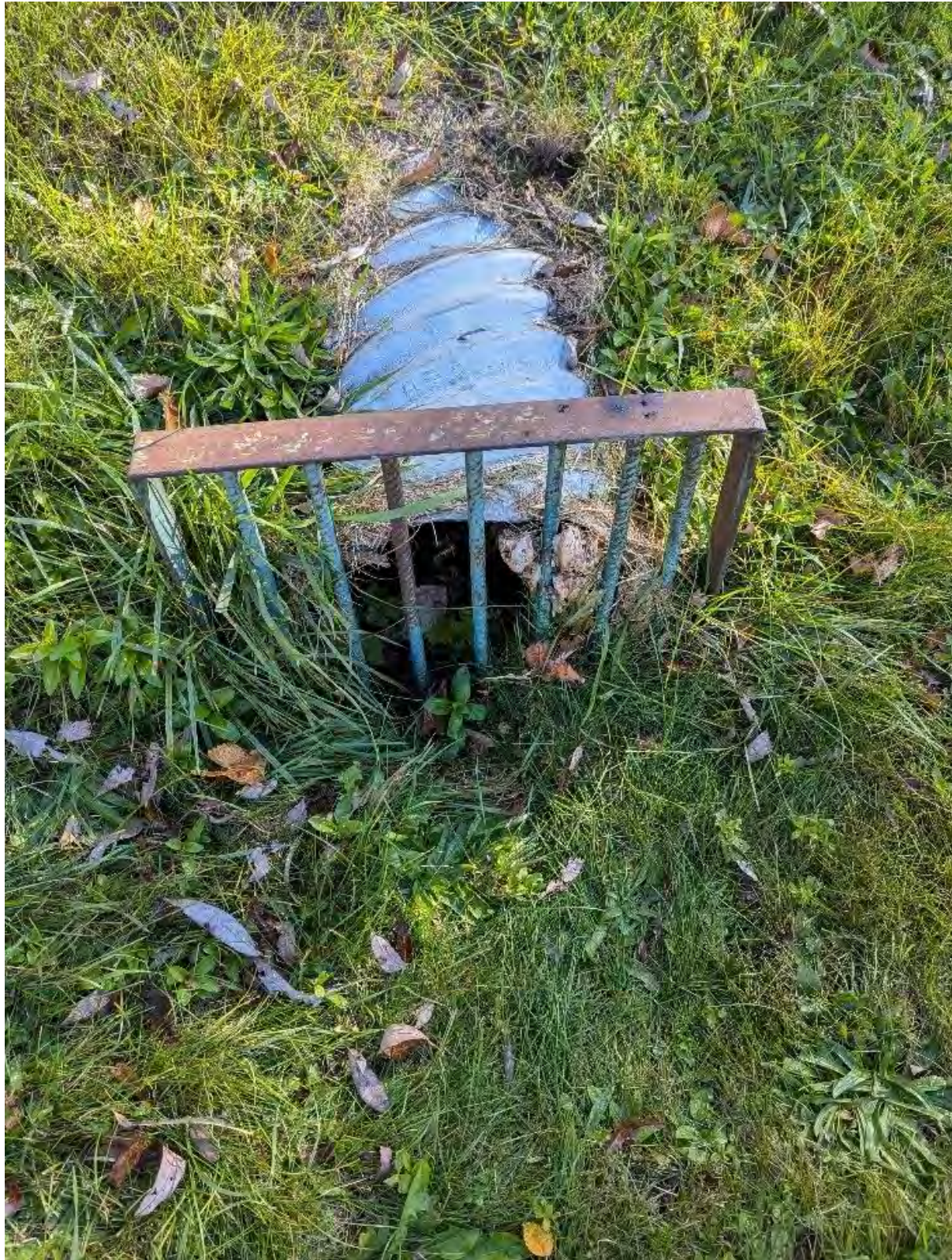
Figure 19: Clear flap gate 1 along Douglas Road berm
