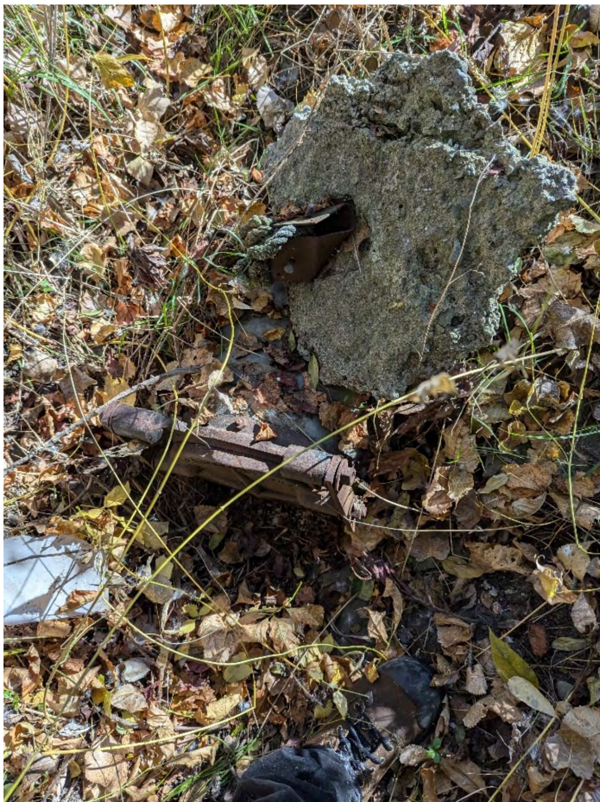
Figure 21: Clear flap gate 3 along Douglas Road berm
