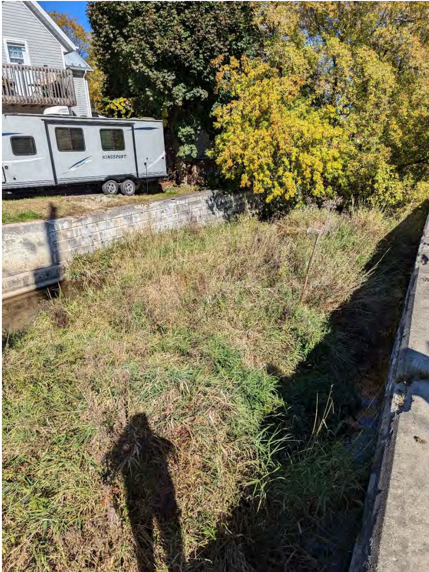
Figure 47: Sediment deposits and vegetation near Simpson Street Bridge and spalling of DuraHold blocks on north side
