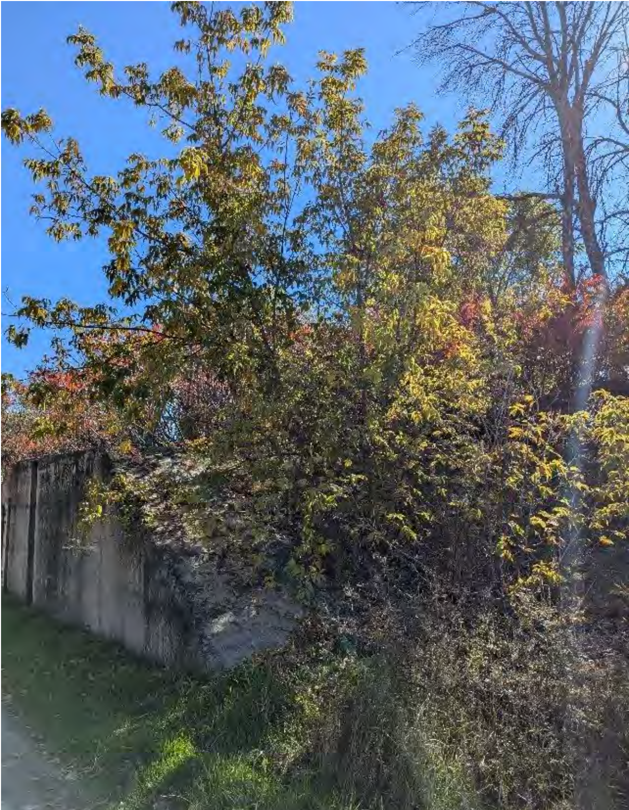
Figure 12: Woody vegetation growth on east side of spillway opening to golf course
