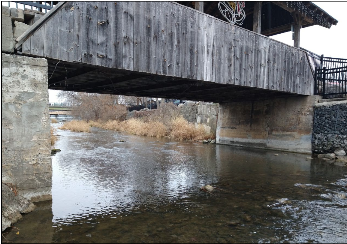
Figure 5-21: Image of Bridge Opening for Pedestrian Crossing Between James St and E Front St.
