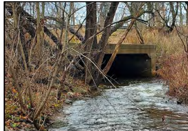
Figure 5-6: Elevation View on Upstream Side of Main Street Concrete Open Footing Box Cu
