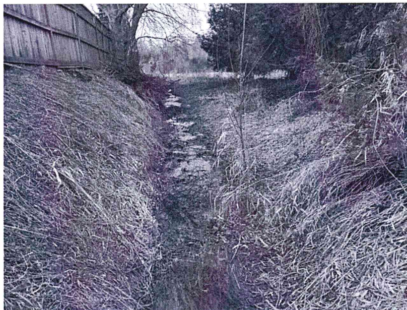
Photo 4 Downstream view of Reach 2: channelized watercourse (from culvert at southeast corner of Site), February 21, 2023.
