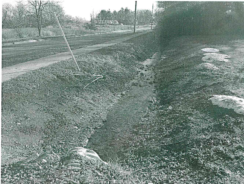
Photo 18 Downstream view of watercourse off-Site along Kensington Ave, December 3, 2021.
